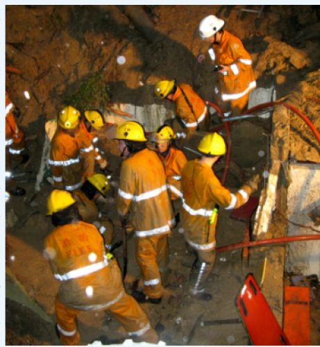
● 消防人員在咖啡灣山泥傾瀉現場拯救被困人士 Fire personnel conducting a rescue operation at the scene of a landslide in Tuen Mun during the black rainstorm
